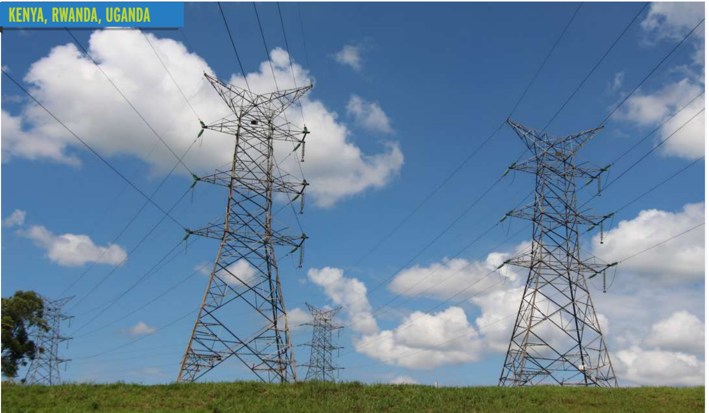
THE KENYA (LESSOS) - UGANDA (TORORO - BUJAGALI) OVERHEAD TRANSMISSION LINE
